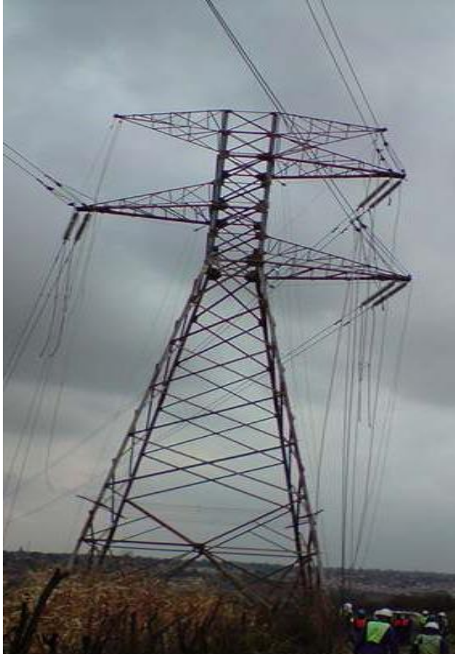
275kV SELF SUPPORTING STRAIN TOWER-422V
